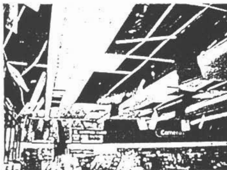
Fig. 12. Thrifty Drug Store — T-bar ceiling with panels displaced and fallen out.
