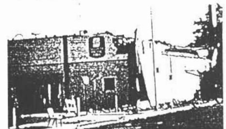
Fig. 9. Old, unreinforced masonry building — Security Pacific Bank — note parapets fallen off.
