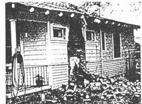
Fig. 16. Unreinforced brick masonry peeled away from the house; no ties.
