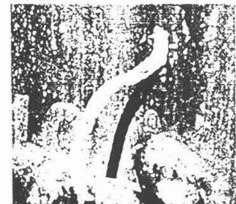
Fig. 17. Corrugated metal ties did not hold the stone veneer in place.
