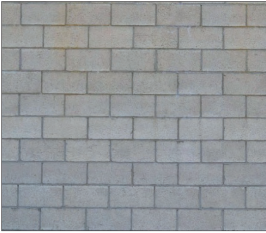
Figure 5 Acceptable CMU wall viewed in diffused light from a minimum of 20 feet away as required by ASTM C90
